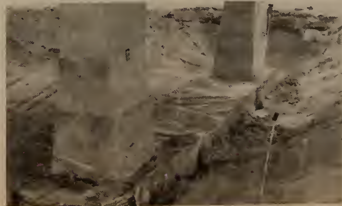
The beginning of excavation for Casey Highway underpinning in the Forest Hills Station area.
